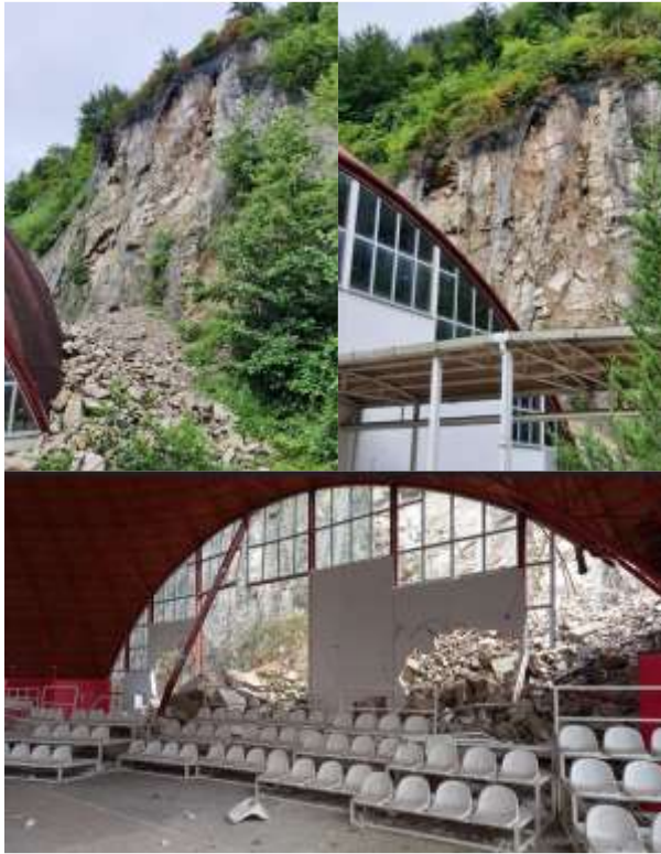
Figure 2: The Hemşin (Rize) rockfall case: the source rock slope and the affected sports facility (top), and the blocks that entered the building (bottom)
