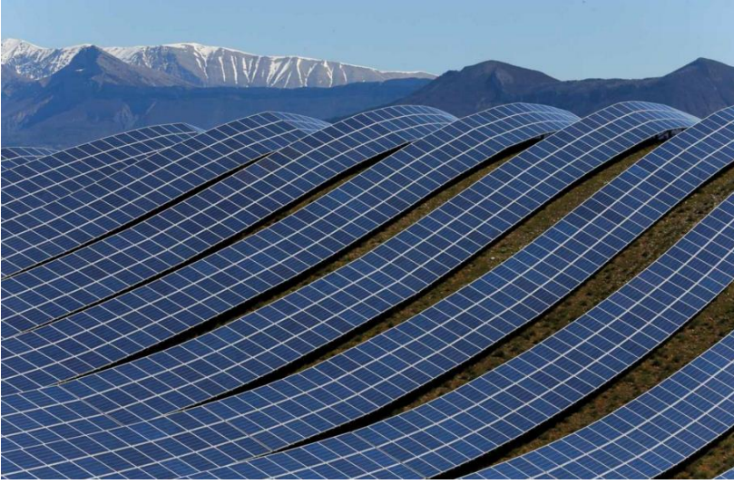
Figure 1. Solar energy system installed on the hills [8, 9]
