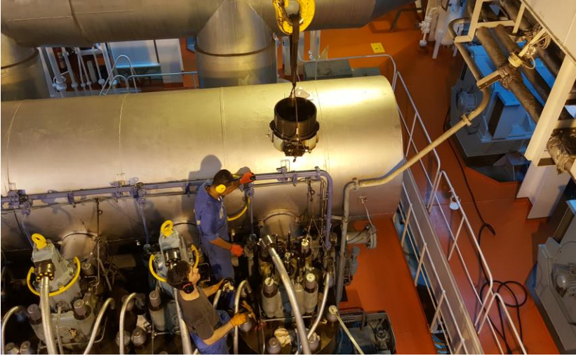
Figure 7: Main engine maintenance
