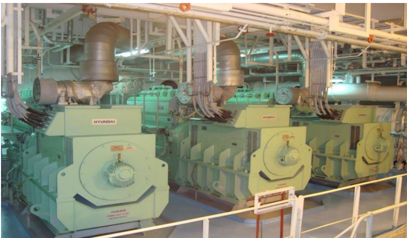
Figure 6: Ship diesel generators
