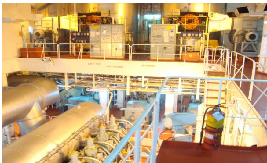
Figure 5: Ship engine room
